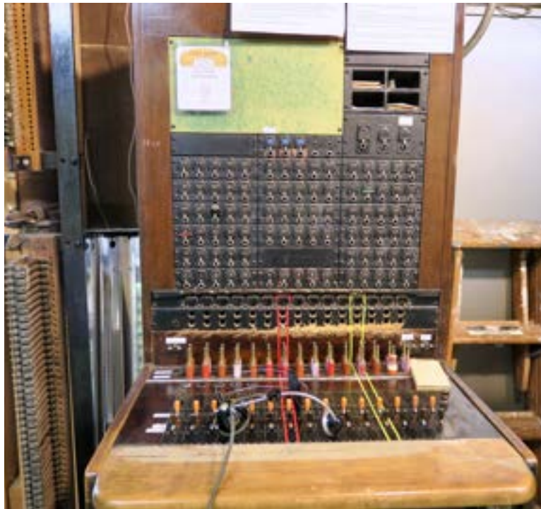
A working magneto switchboard in the collection of The Telephone Museum in Ellsworth.
